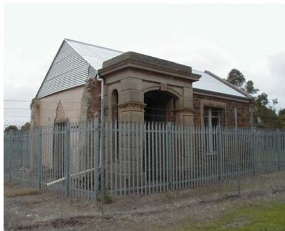
Lochend House, in Campbelltown SA, in the early stages of restoration. Note that one of the two front rooms had been completely demolished.
